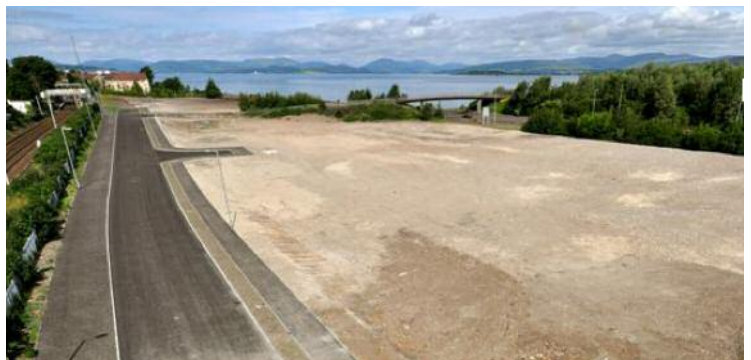
The 30,000 square metres site at Kelburn, platformed and ready for light industrial use
